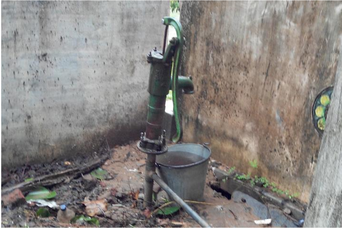
The house's water supply (before)
