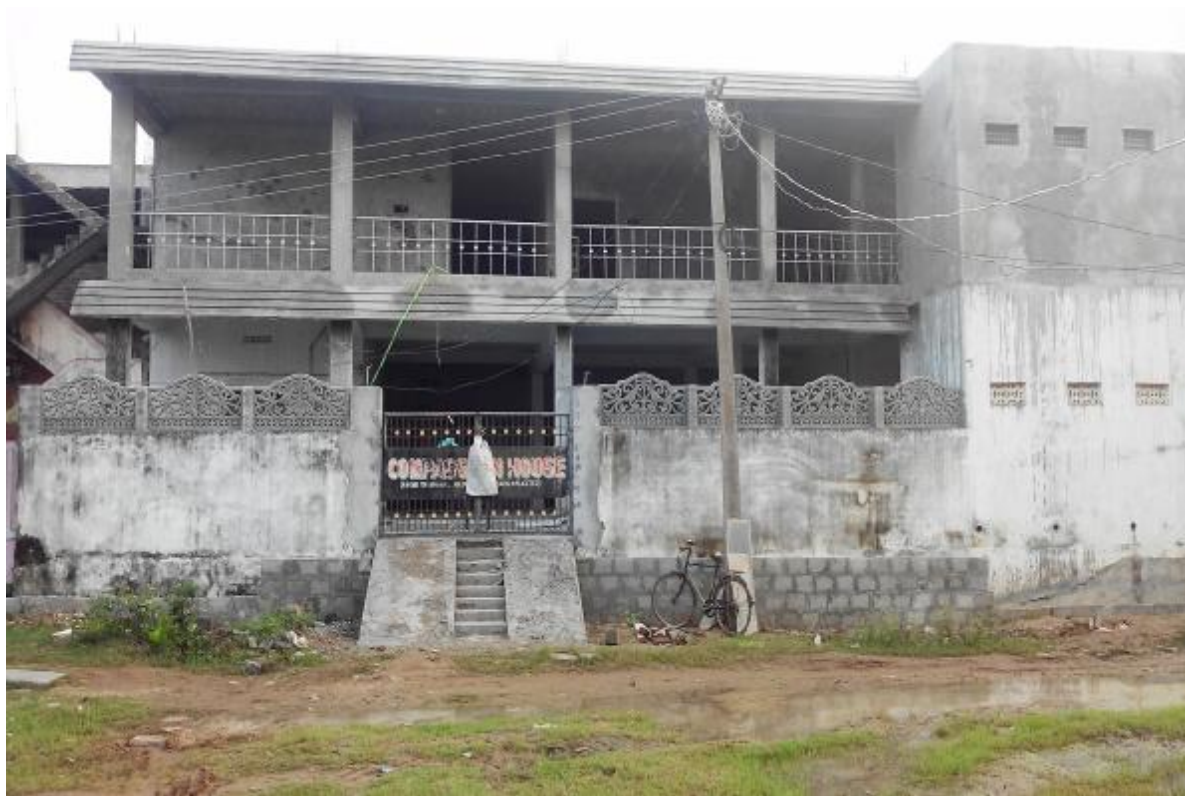
The front gate to the Compassion House (after) still more to be done
