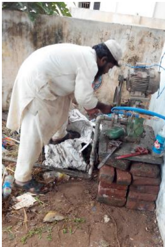
The new water pump
